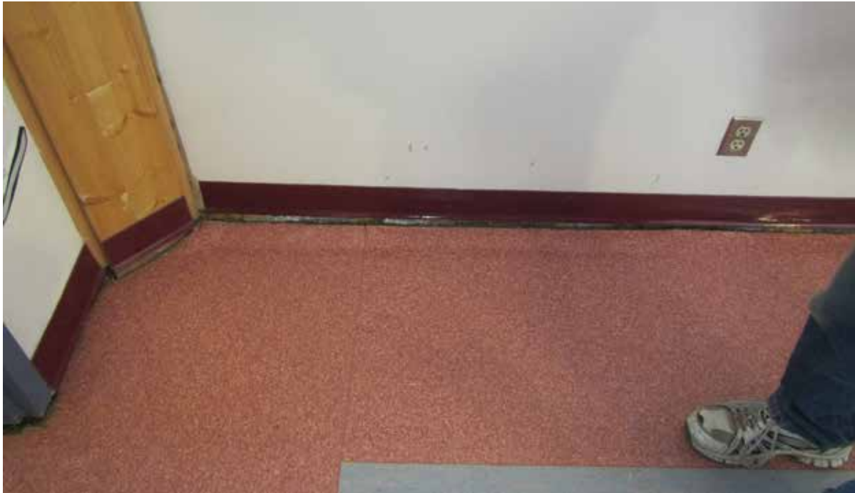
Figure 4.1.3 Gaps in joints between walls, and between walls and the floor, school
