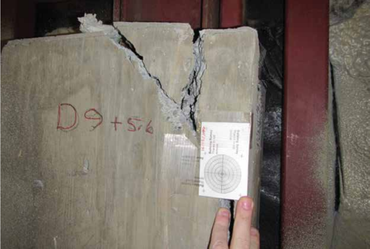
Figure 2.7.1.2 Damage to a concrete pier in the southwest part of the school
