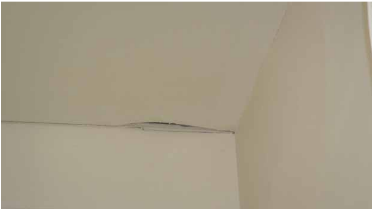
Figure 4.1.4 Small cracks between walls and ceiling, community centre
