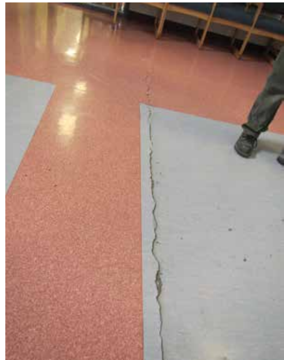
Figure 4.1.2 Cracks in the floor, school
