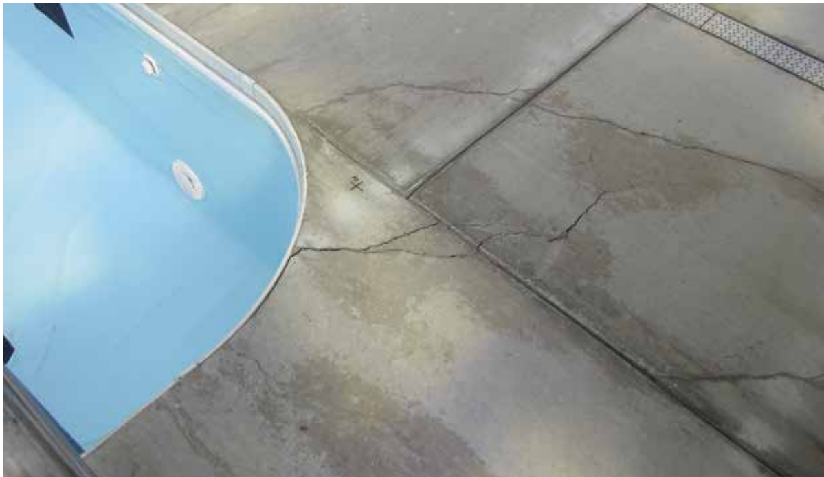
Figure 4.1.7 Cracks in concrete floor, pool
