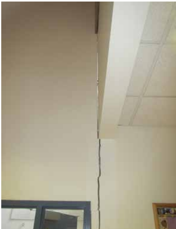
Figure 4.1.1 Cracked drywall, school
