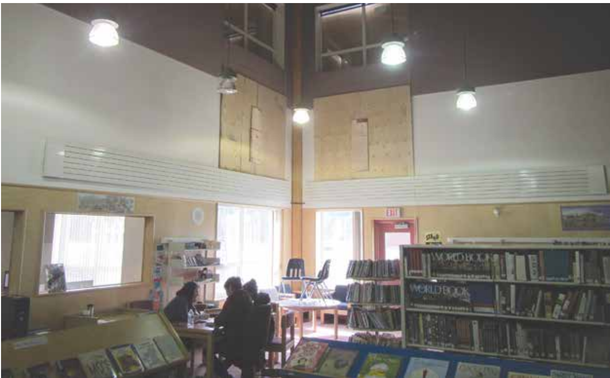
Figure 4.1.6 Window glass replaced by plywood, school
