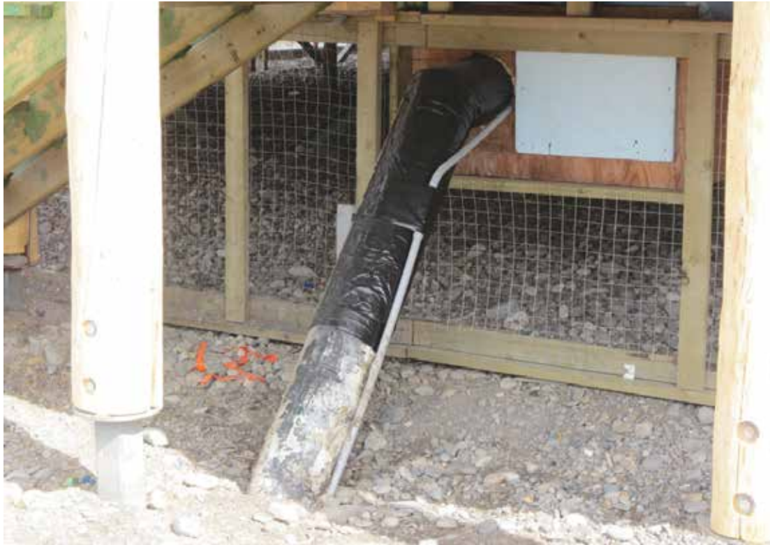
Figure 2.7.2.1 Repaired sewer line; sewer line had leaked for an unknown amount of time
