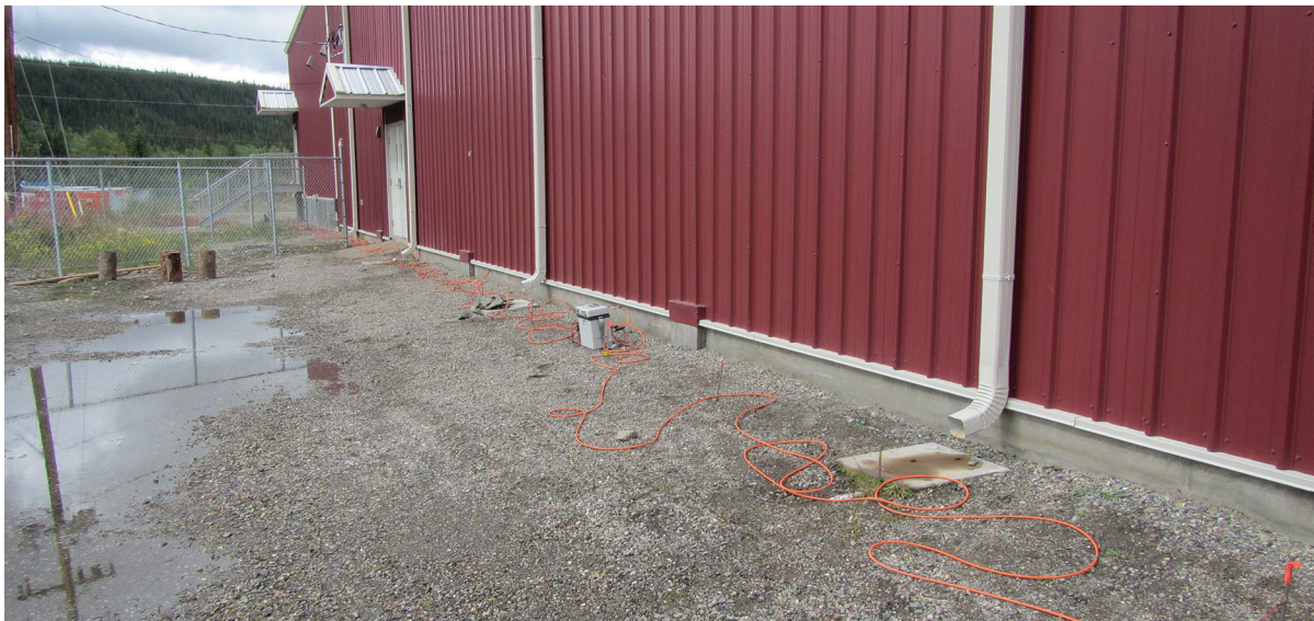
Figure 5.2 Water accumulation at the south side of the arena
