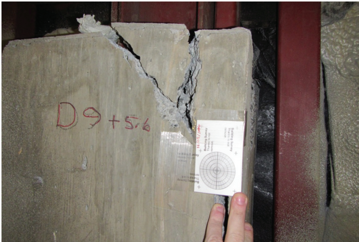
Figure 2.7.1.2 Damage to a concrete pier in the southwest part of the school
