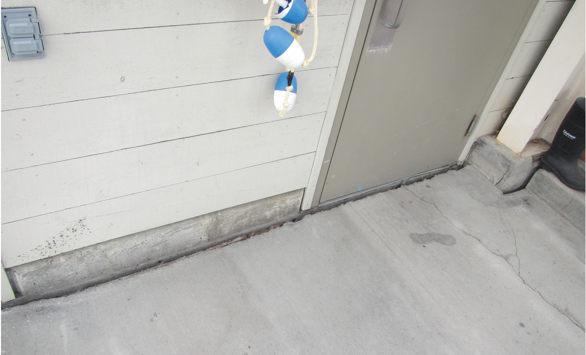
Figure 4.1.5 Gap between the wall and the floor, pool
