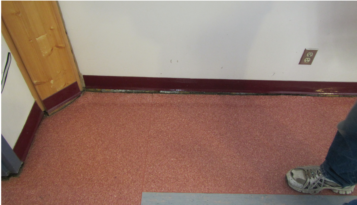
Figure 4.1.3 Gaps in joints between walls, and between walls and the floor, school
