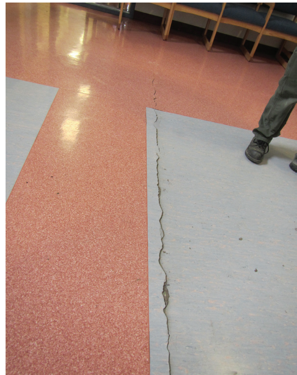
Figure 4.1.2 Cracks in the floor, school
