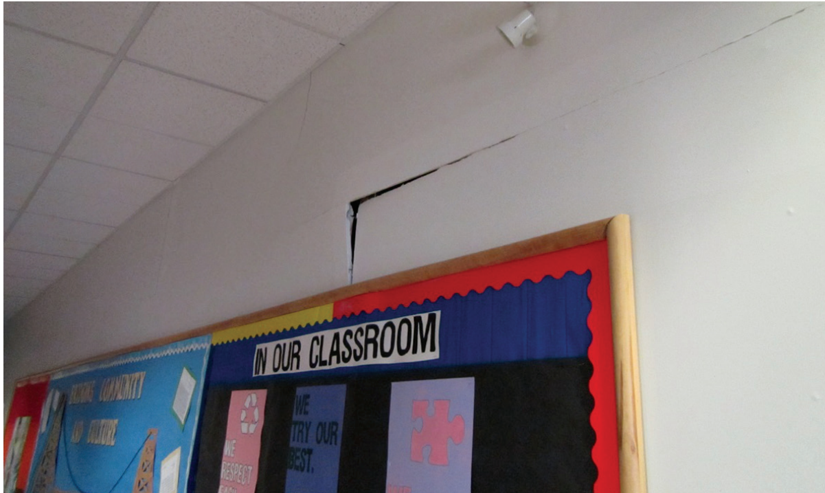
Figure 2.7.1.1 Damage to drywall in the northeast part of the school
