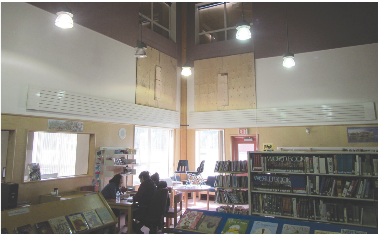
Figure 4.1.6 Window glass replaced by plywood, school
