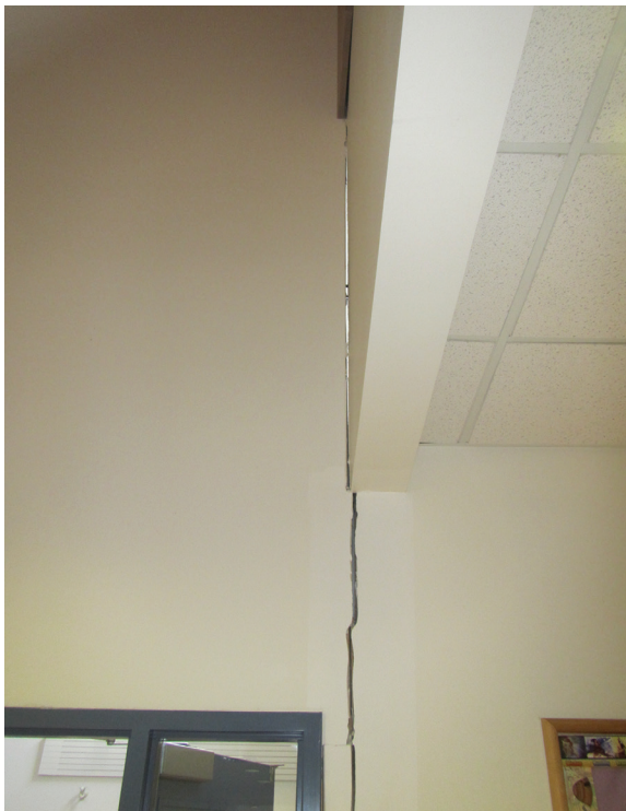
Figure 4.1.1 Cracked drywall, school
