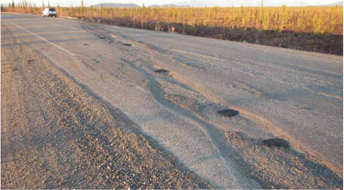
Degradation observed at km 1881.
