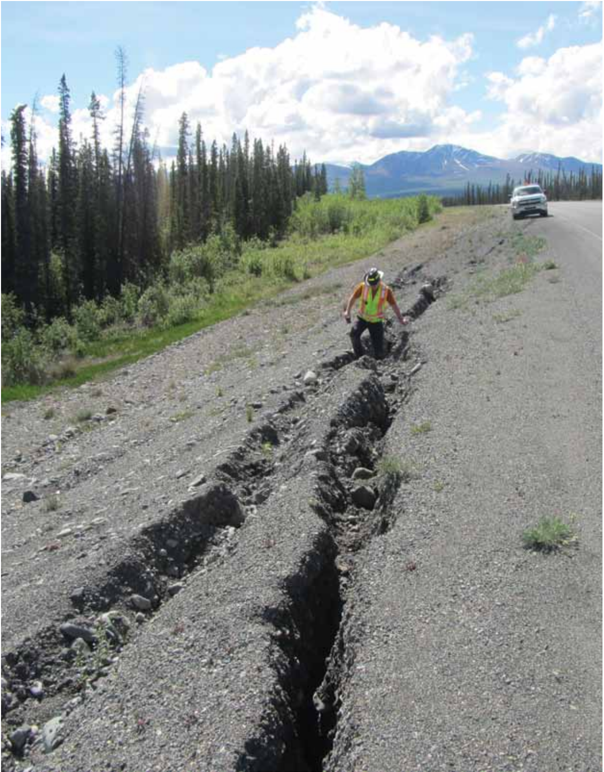
Longitudinal cracking observed at km 1713.
