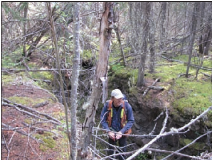
Figure 20. An example of the largest tension crack observed in point bar sediments deposited by the Stewart River. This crack is ~1.5 m deep and can be traced for more than 500 m.
