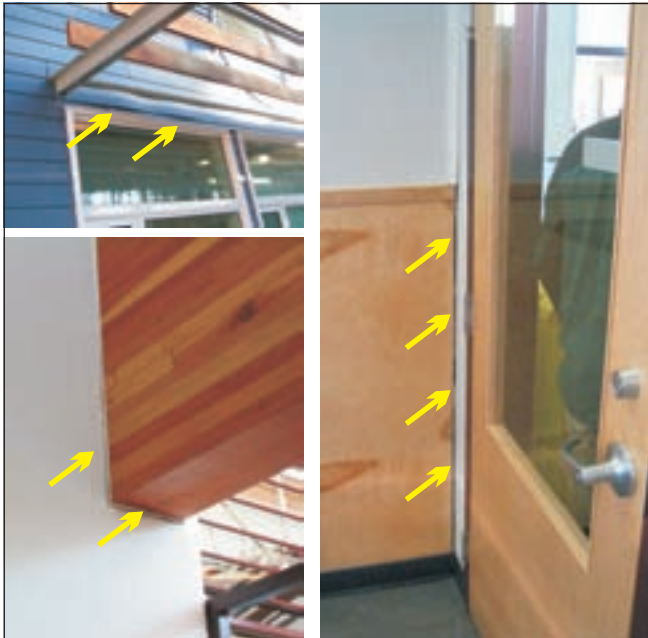
Figure 25. Examples of infrastructure damage due to permafrost thawing and ground subsidence observed at the Yukon College annex, J.V. Clark School, Mayo.
