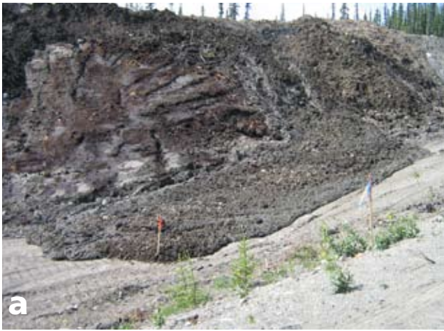
FIG 2.4 a: Melting permafrost. Ice-rich ground was encountered unexpectedly during slope work at this road reconstruction site. The disturbance and removal of insulating ground cover caused thermal destabilization of the ice and initiated melting. The debris flow in the foreground is sediment saturated with water from the melting ice. Once initiated, such melting is difficult to halt. If ice bodies in permafrost ground are disturbed, the situation should be remediated as quickly as possible with the application of granular fill, organic materials and a dense seeding of grasses adapted for cold, wet soils (it is important to measure the pH of these sites and match the grass species accordingly).
