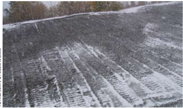
(f) This slope has been properly trackwalked. Notice how the tractor was driven up-slope, rather than cross-slope. The result is that cleat tracks run perpendicular to the slope and serve as catchments for seed, fertilizer and surface water.
