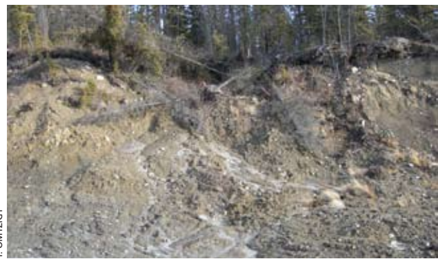
(j) Revegetation cannot be used to solve every slope issue, at least not alone. This slope is slumping for two reasons. First, the slope was cut at a steep angle into unconsolidated fill (glacial till) that is difficult to stabilize. Second, the situation is aggravated by the presence of a small drainage that runs off onto the newly exposed surface. Solution: control (divert or channel) drainage, decrease the slope angle and consider bioengineering solutions (see Chapter 4). Only then will the surface be stable enough for seeding.
