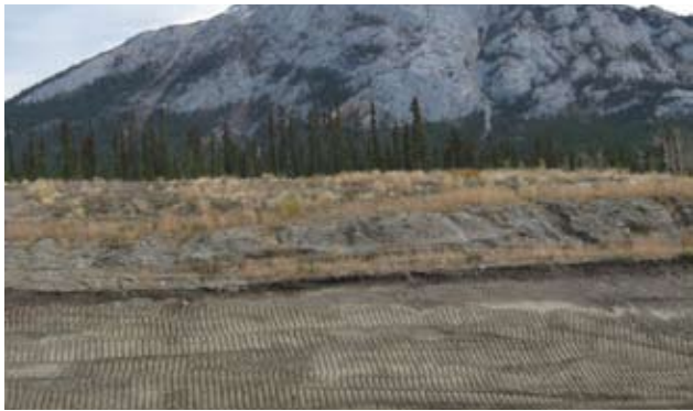
(g) This slope has not been properly trackwalked. The tractor was driven across the slope leaving cleat tracks running parallel to the slope. Surface water will run down these tracks causing rill formation and loss of seed and fertilizer due to runoff.
