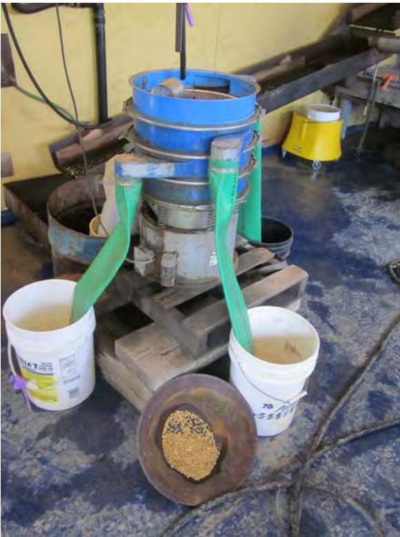
Figure 28 - Left - Sweco Rotary Screen for Splitting Secondary Concentrates in Various Size Fractions – The coarse fraction for hand picking, medium and fine fractions for processing on the Gold Wheel possibly followed by processing on a Shaking Table.
