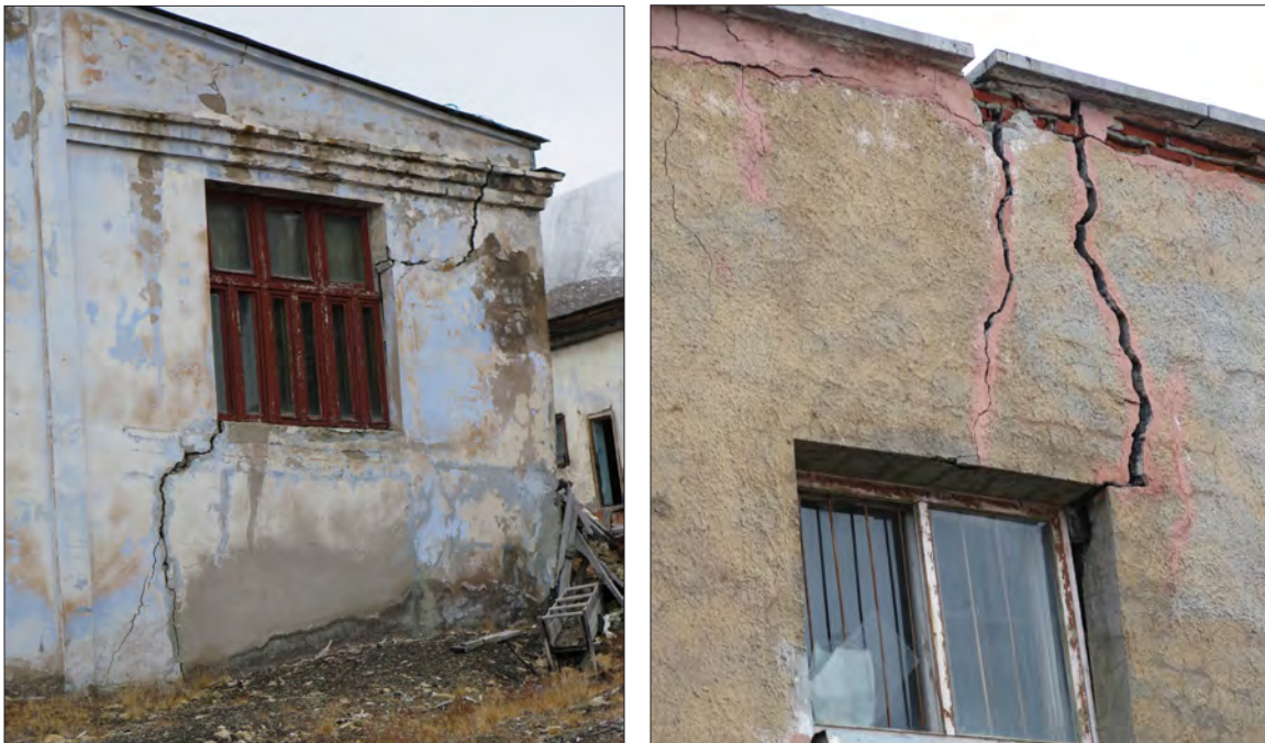
Figure C3. Examples of unmaintained buildings in Pyramiden, Svalbard, displaying cracks and uneven settlement in response to permafrost thaw.
