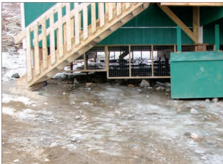
Figure C18. Example of water ponding around a foundation built on permafrost (Government of Nunavut, 2013). Water ponding can have a negative impact on permafrost thermal regimes.
