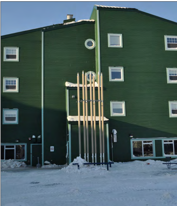
Figure C16. Example of thermosyphons, a foundation system that requires a significant amount of expertise to design, install, maintain and monitor (CSA, 2014).
