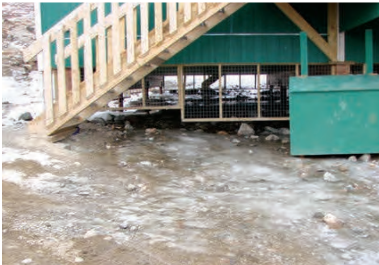
Figure F18. Example of water ponding around a foundation built on permafrost (Government of Nunavut, 2013). Water ponding can have a negative impact on permafrost thermal regimes.
