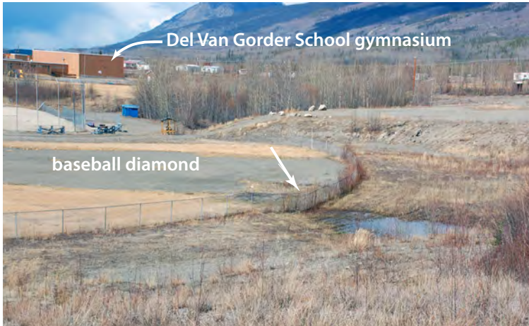
Figure 40. Surface settlement (indicated by white arrow pointing to a dip in the fence line and adjacent ponding) at the Faro baseball diamond is likely caused by permafrost degradation. Photo: Kenji Yoshikawa, 2007.
