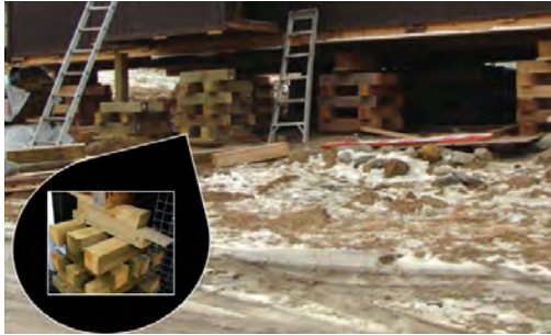
Figure F12. Example of a timber-block foundation used in Nunavut (Government of Nunavut, 2013).
