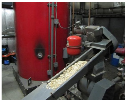
KFN's wood chip boiler. JP Pinard.
